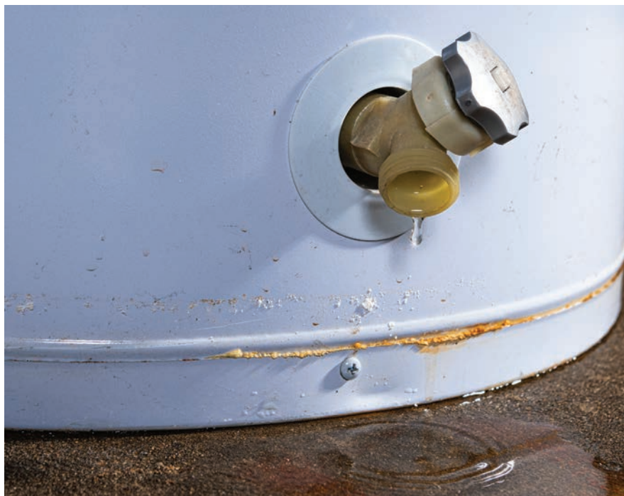
Mineral buildup at the bottom reduces efficiency and can cause the tank to overheat and fail prematurely.
